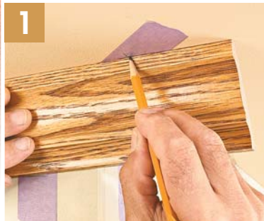
1 ▲ Locate Upper Corner To locate the upper outside corner of two adjoining moldings, mark along the top edge of each piece, forming intersecting lines.
